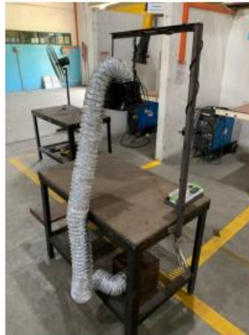
Figure 1. Exhaust Fan with Smart Gas Detector
